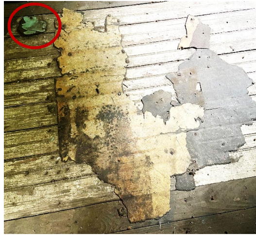
Figure 14b: Remnants of vinyl floor tile in the Ailey Young House
