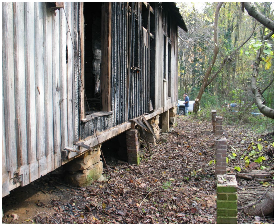
Figure 4: Photo of the south side of the Ailey Young House. Taken in November 2009 showing the remains of the brick piers and deck boards for the front porch.
